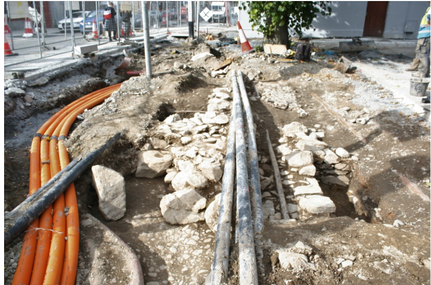
Church of Ireland facing north, showing new pipes to west of wall C140
