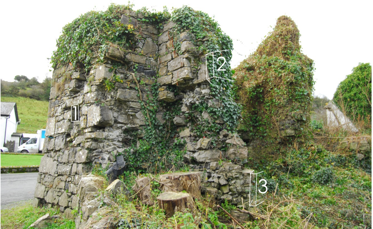
View of east face of building showing: 1 - staircase arrow loop, 2 - upper floor arrow-loop, and 3, ground-floor arrow-loop
