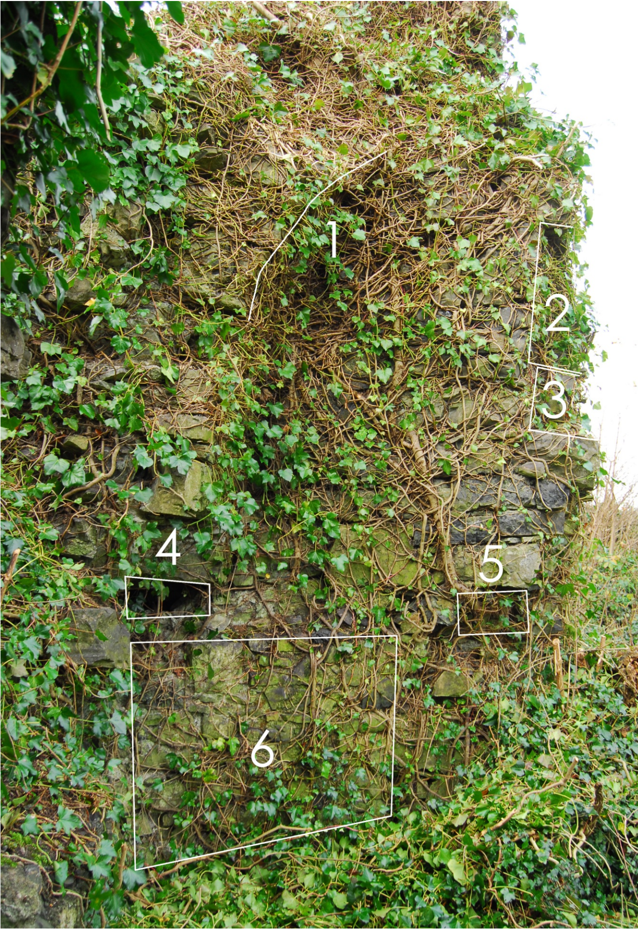
Internal western wall facing west showing: 1 - curve of chimney stack, 2 - upper floor fireplace opening, 3, putlog hole for beam holding up upper floor, 4 & 5 - holes to hold up possible mantle piece at ground floor, 6 - protruding masonry relating to ground floor fireplace
