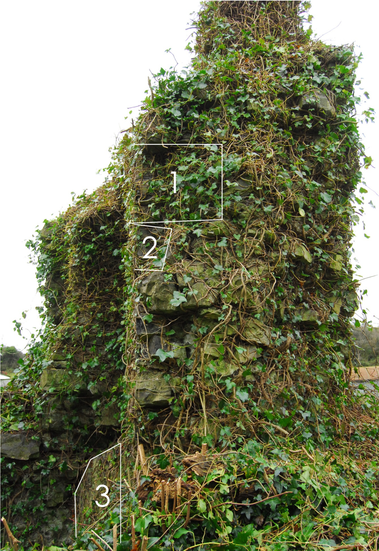
Western wall facing north showing: 1 - upper floor fireplace opening, 2, putlog hole for beam holding up upper floor, 3 - protruding masonry relating to ground floor fireplace
