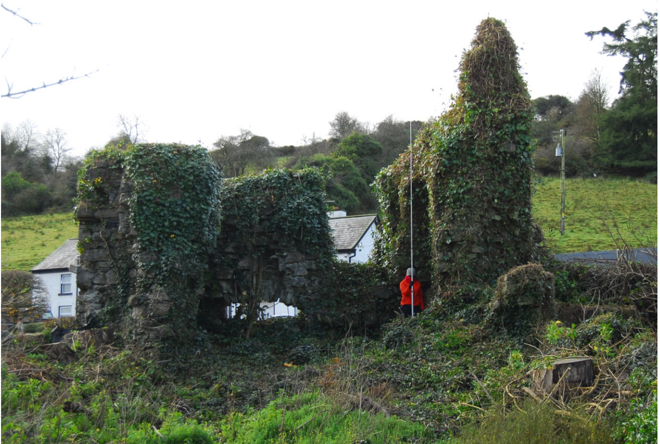
View of rear of building, facing north, showing interior and absence of southern (back) wall
