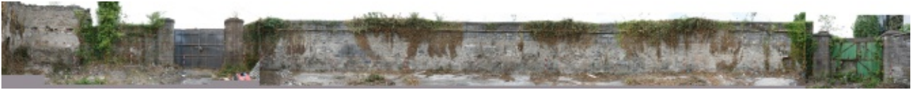
Scaled and rectified photographic elevation of southern boundary wall (internal), overlaid with 1m orange grid. Refer overleaf for closeup.
