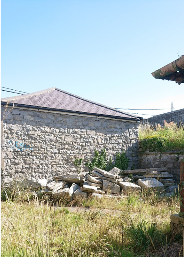
Pile of loose granite south of Building E Wagon shed
