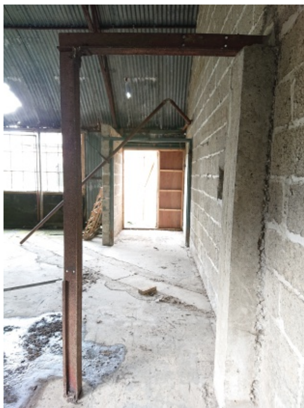
Paxo Plant Building B, showing concrete-roofed drain under floor drain and steel frame near wall hatch
