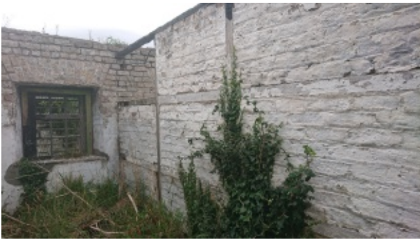
Building D showing unusual construction of brick and timber late 19th century wall, mirroring Building F.
