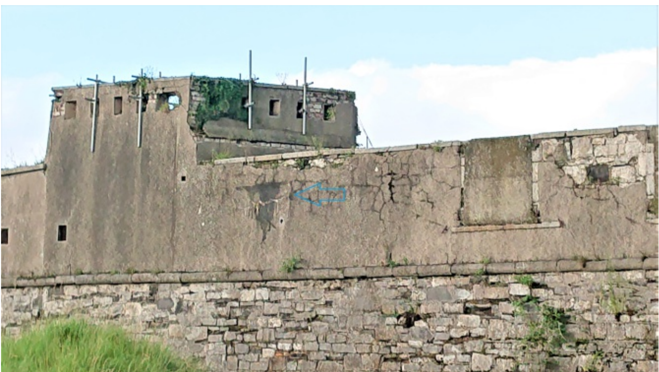
Exterior of rampart wall showing repair north of Cavalier 1, mentioned by Buggle in 1936
