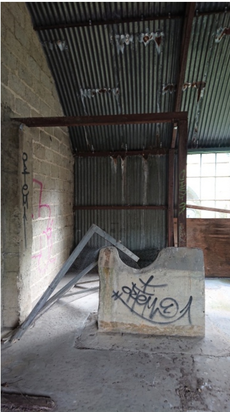
Paxo plant building B showing unidentified machinery base, possibly for a grinder. Traces of the per-1940s steel wall removed for the Paxo Plant are visible in the floor in the right foreground
