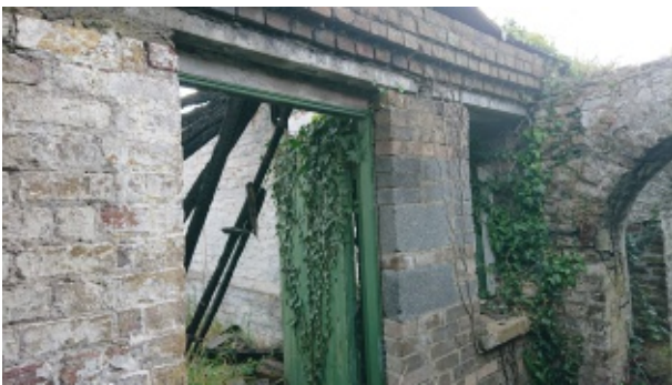
Building D showing reinforcement of doorways, possibly related to additional security and repair following 1916
