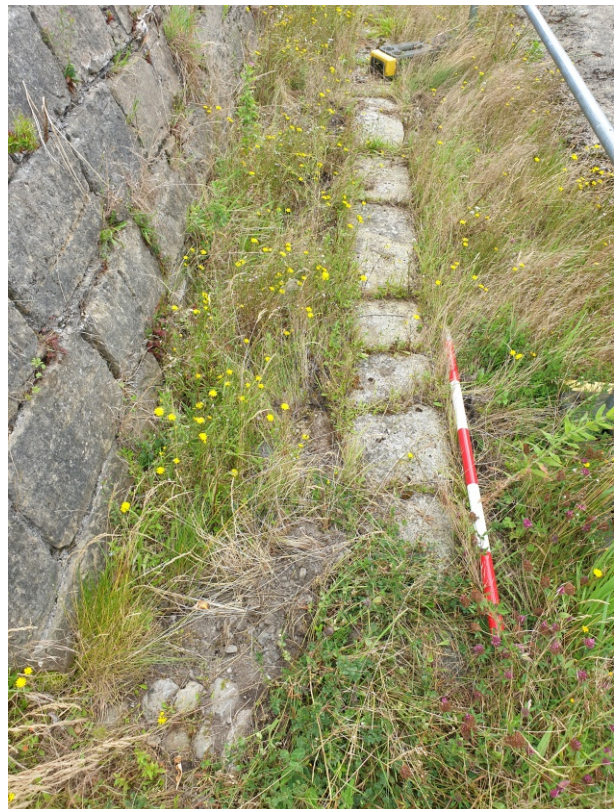
Granite 'sentry promenade' to west of Blast Wall in main fort. Note abrupt end of cobbles at base of image indicating missing upper step
