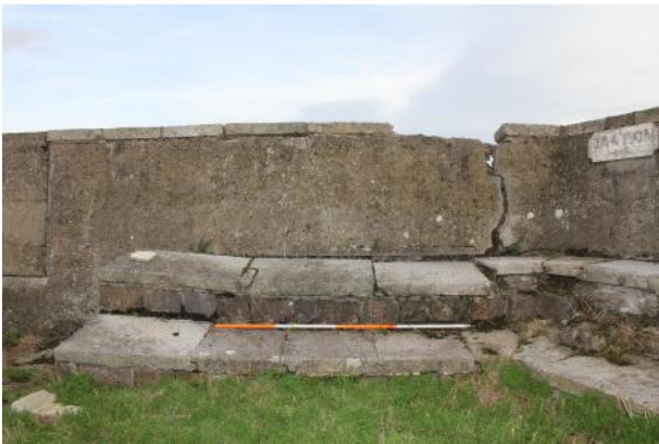
Rampart walkway to S of gun emplacement. Note substantial subsidence of steps under the crack in parapet wall.
