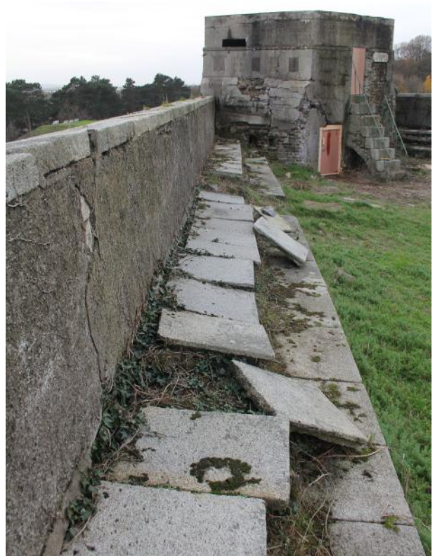
Looking W along the S wall of the SW bastion. Note collapsed granite walkway slabs.
