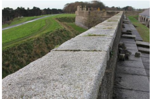
Looking W along the granite capstones of the parapet wall in Area A.
