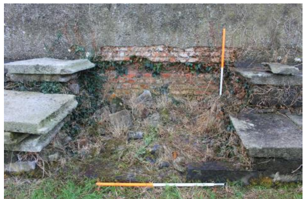
Breach in parapet walkway. Note slot in brick section of parapet wall created to hold granite slabs.
