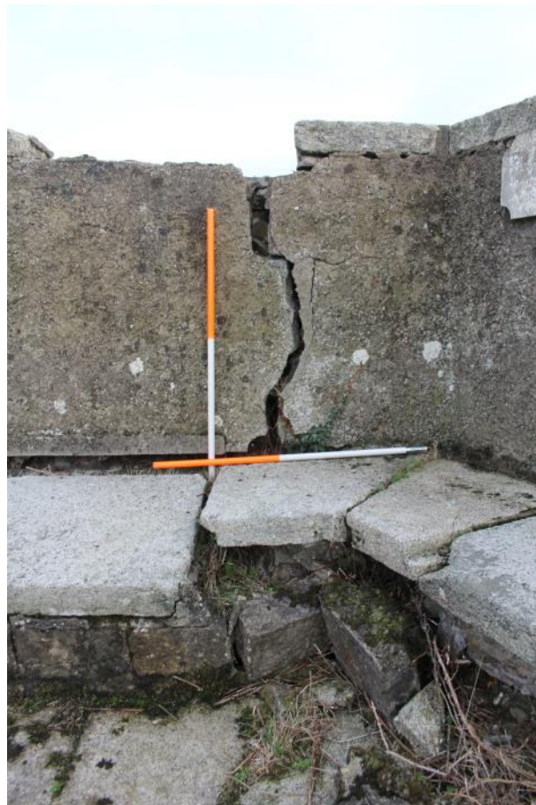
Detail of major crack in SE corner of W-facing wall of bastion.
