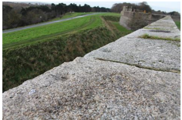
Oblique view of small indentations along outside edge of granite capstones on the parapet wall. Looking W.
