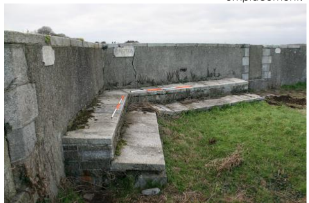
Detail of walkway at SW corner of NW bastion as it runs between the two gun emplacements.
