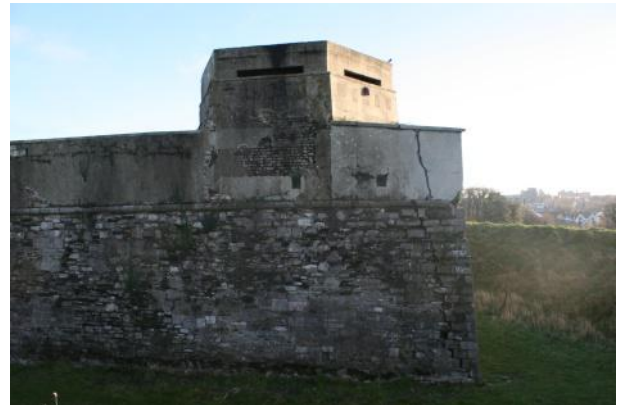
Area B, SW cavalier looking E Note major crack.
