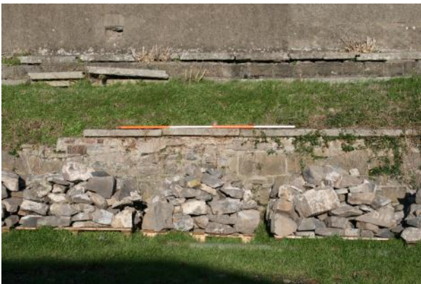
Detail of S-facing rampart retaining wall. View of the wall is obscured by piles of cut stone.
