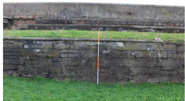
Rampart retaining wall at E end of Area A. Note regular coursing.
