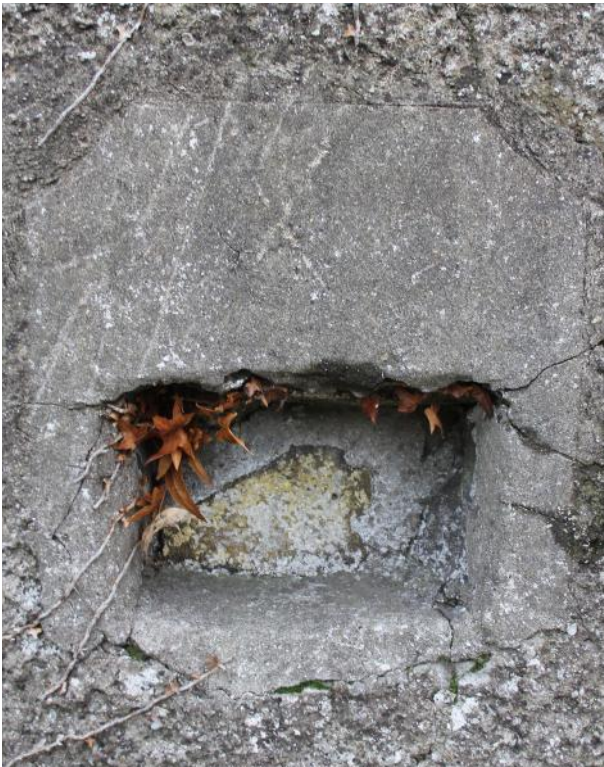
Detail of rectangular cement-lined niche at W end of S wall of bastion.
