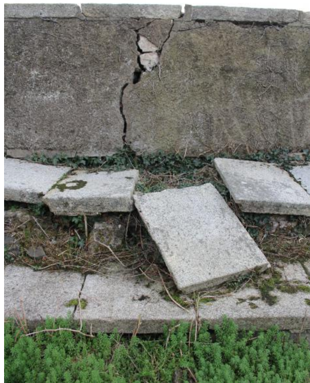
Detail of major crack in E end of S wall of bastion. Note collapsed walkway slabs under crack.
