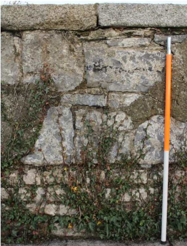
Detail of parapet wall stripped of pebbledash on N wall of SE bastion. This is outside but close to Area A.
