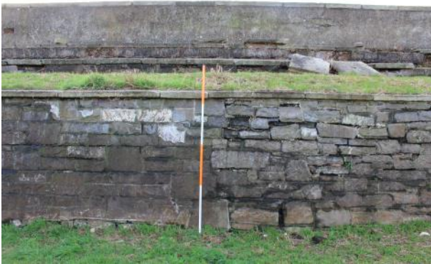
Rampart retaining wall in at W end of Area A. Note junction between coursing styles.
