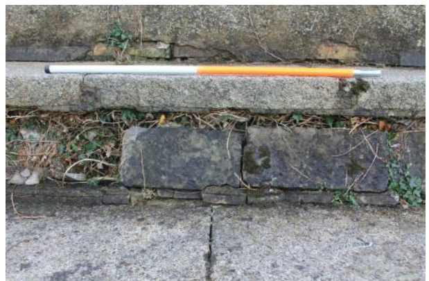
Detail of riser of upper step. Note how cement has been used to fill gap created by subsidence.
