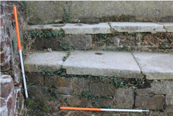
Junction of SE cavalier and stepped rampart walkway. Note facing of step risers.
