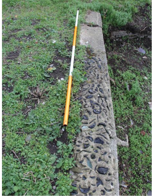
View S along W-facing rampart retaining wall showing cement and glass layer above capstones.
