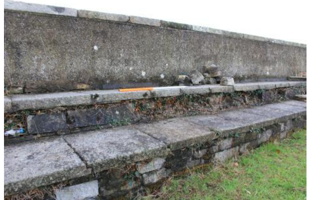
View of rampart walkway mid-way along Area A. Note collapsed facing stones on upper riser.
