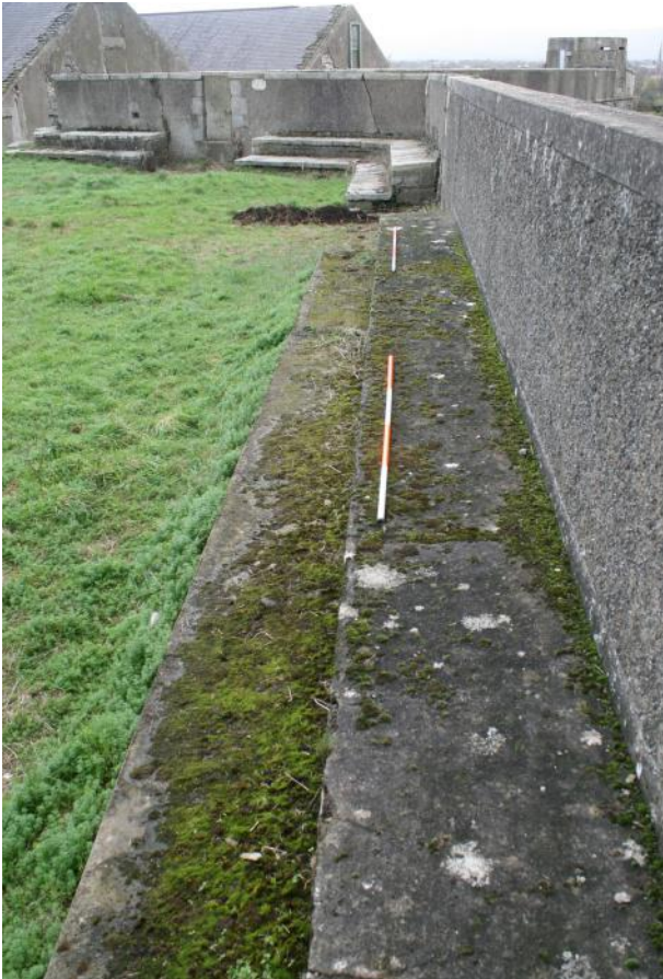
General view of stepped walkway in NW bastion looking SE from NW cavalier.
