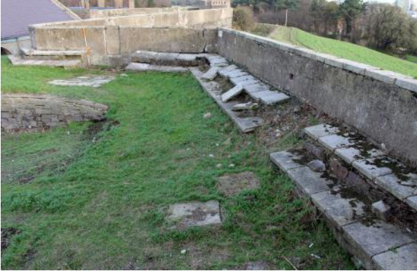
View across Area B from SW cavalier showing stepped walkway. Looking E.
