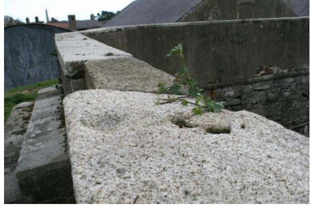
Circular indentations cut into granite capstones at S gun ope. Looking E.
