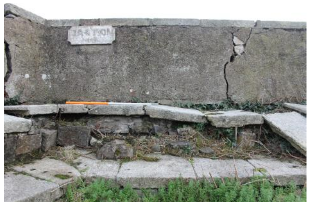
E end of S wall of bastion. Note subsidence of granite steps and the total collapse of the facing stones of the upper riser.
