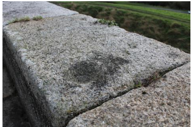
Oblique view of large indentation in parapet wall capstone.
