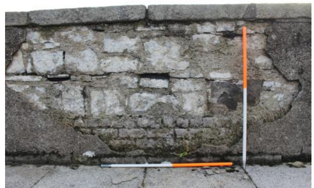
Parapet wall at NW-facing segment of parapet wall. Pebbledash had fallen off here revealing the courses of brick and stone in the wall.
