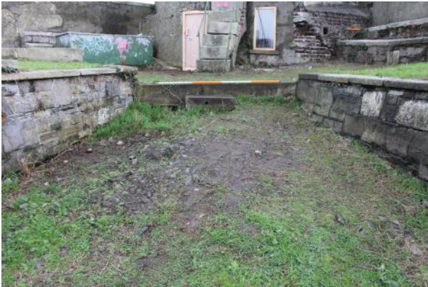
Ramp and concrete step at E end of retaining wall leading to cavalier.
