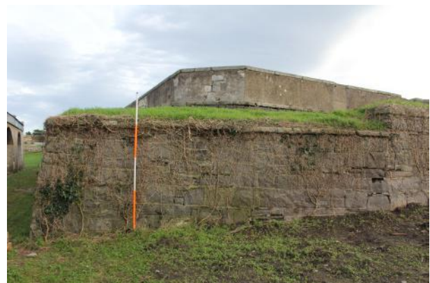
NNW-facing retaining rampart wall. Note batter at N end of wall and step at S end.
