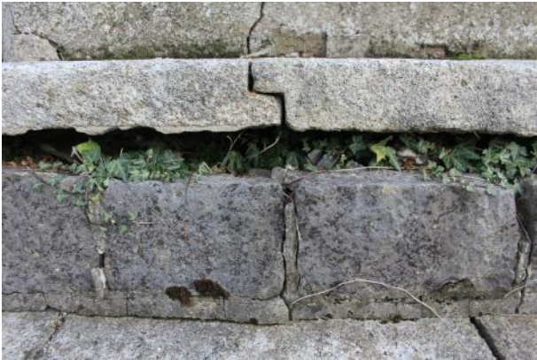
Detail of upper step and riser to N of gun emplacement in Area B. Note joggle on granite slab. Note also large gap between upper slab and facing stones and thick cement pointing along base of risers.
