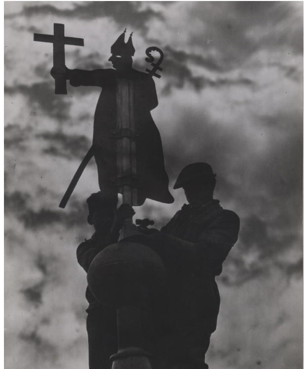
Repairs to the copper roof by Tony Cousins and his uncle Patrick Dorrington in 1958 (Guinness Archives ref GDB.EN02.0003.01 mas)
