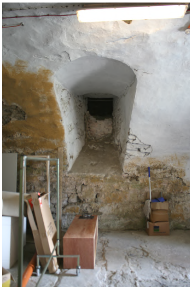
16th century blocked window opening in northeast of basement, missing window frame, showing what 16th century window might have looked like originally prior to the 18th century
