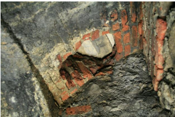
cellar 1 hole in ceiling (for drain)
