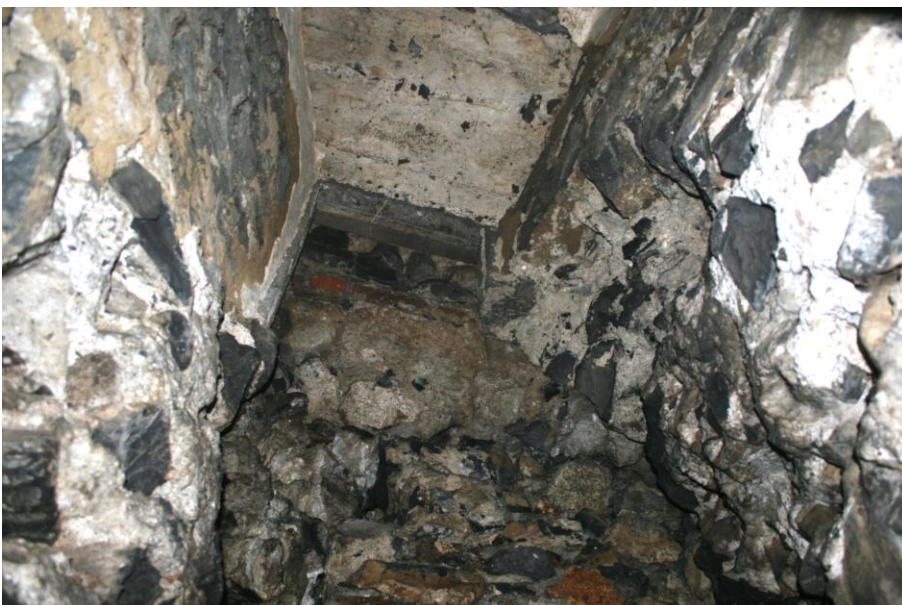
View upwards through hole, showing 16th century window opening and original? stone window frame
