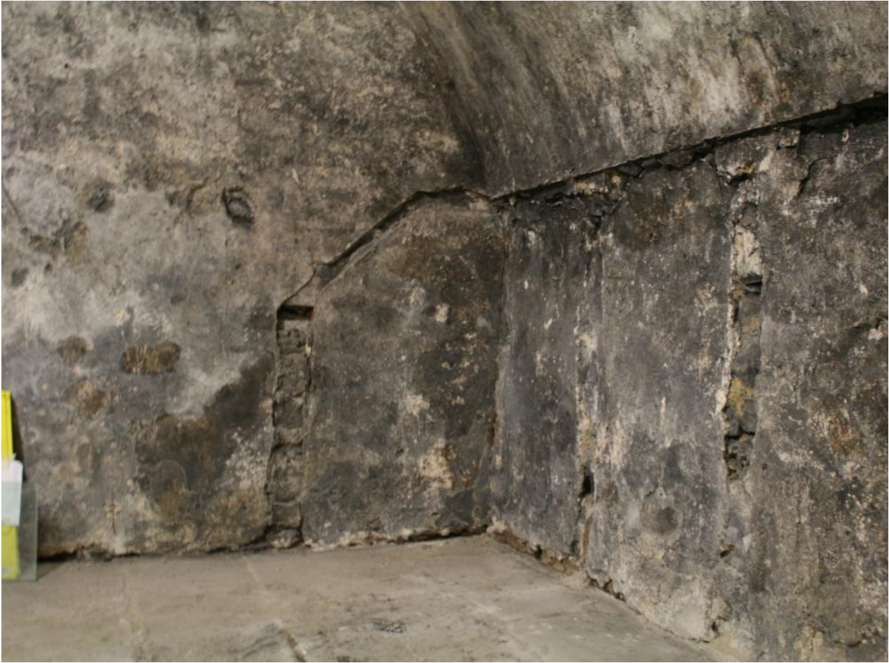
Traces of coal bunkers visible by areas of missing plaster in wall of basement
