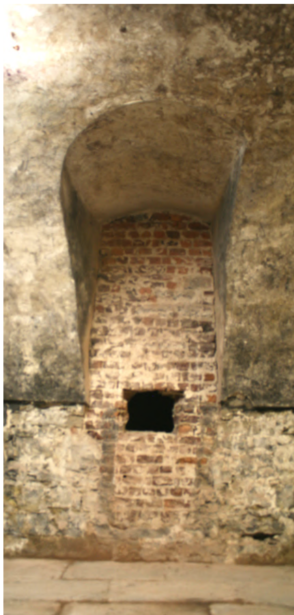
Works area showing hole in wall
