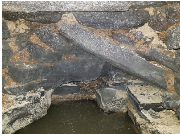
Masonry drain vault as it runs under the spine wall to the castle. this part of the drain dates to 1583
