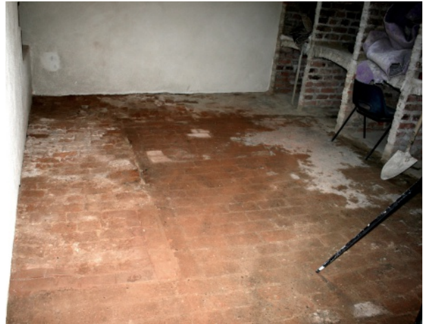
Brick floor in tower B10 following conservation, showing footing of earlier shelves in left of image
