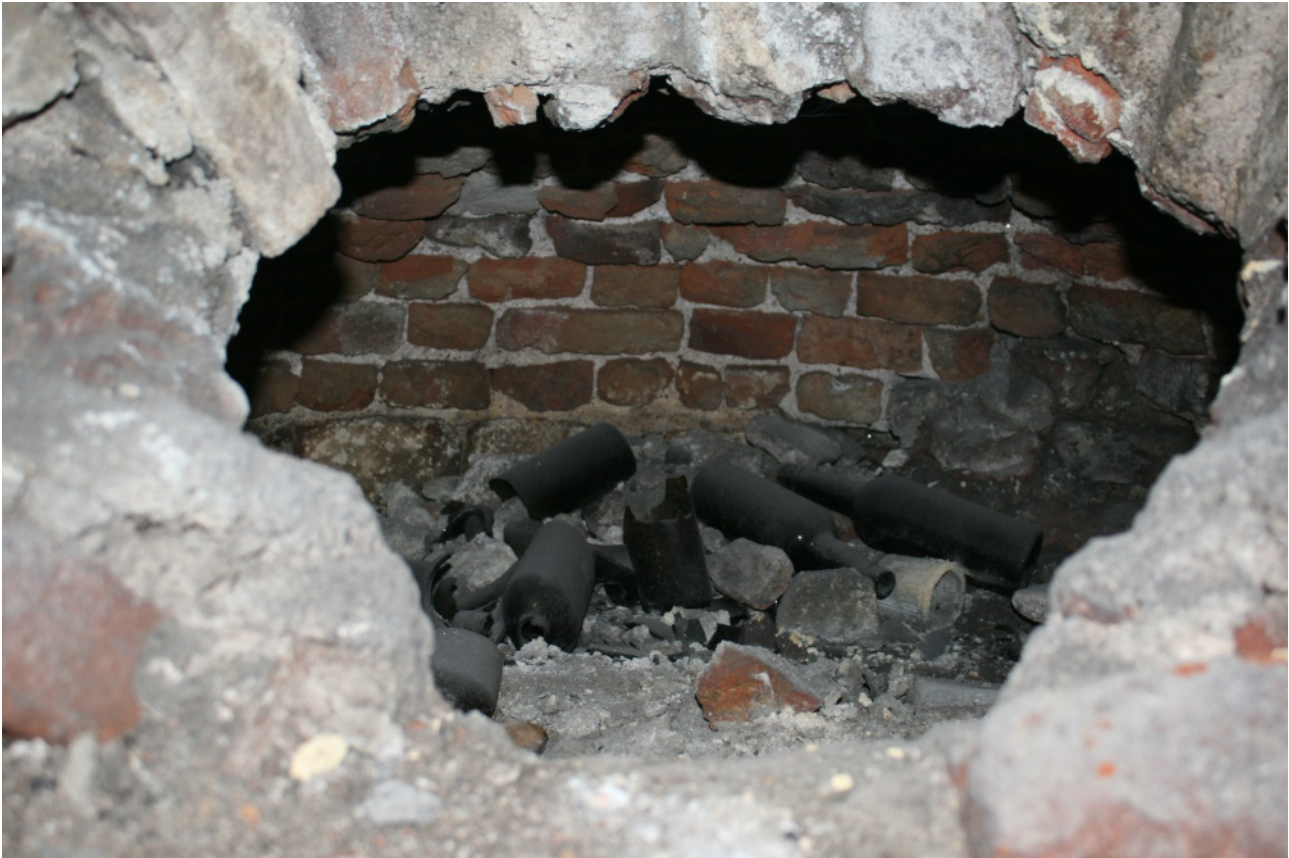
View into bake oven during restoration works, after damaged brick infill was temporarily removed. Visible is a brick oven dome, partially backfilled with demolition rubble, and numerous late 19th or 20th century glass bottles. These were left in situ
