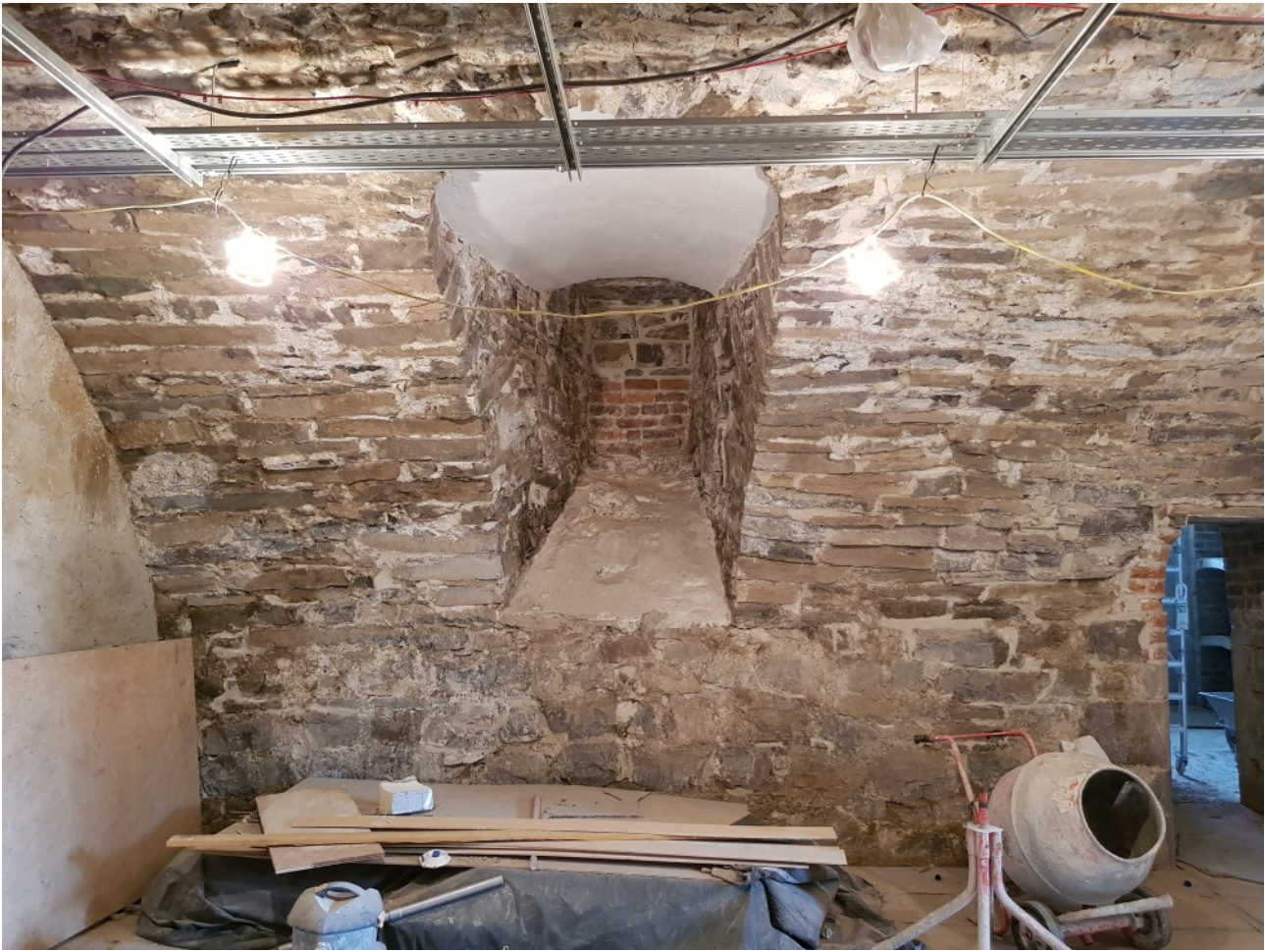
16th century wall surface in Rathfarnham Castle basement. This is the north wall of Room B7
