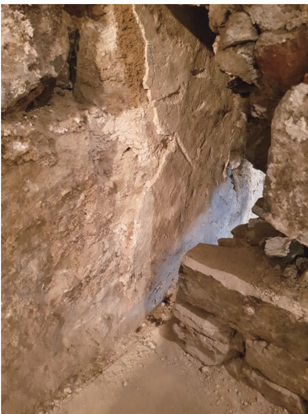
Earth mortar plaster in situ on north wall between B7 and B8, surviving behind the wall dividing the two rooms
