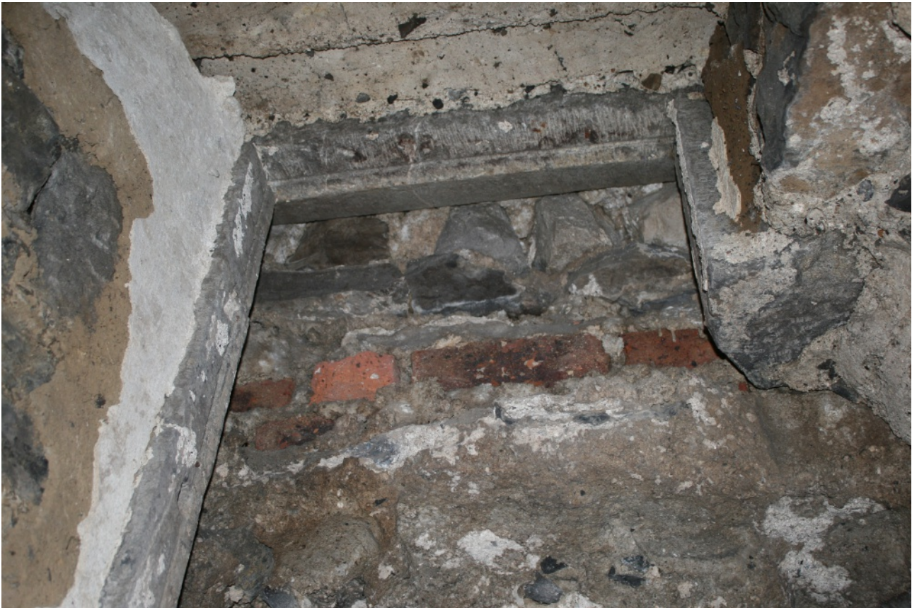
Blocked 16th century window in north wall of castle (Room B8) identified in 2016. Note type A earth plaster over stone window frame on right of embrasure
