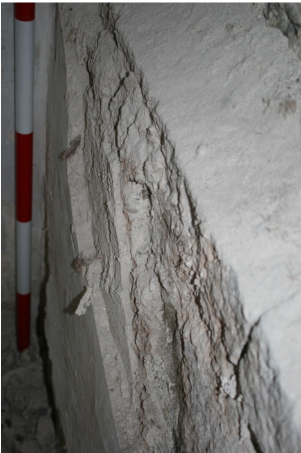
Possible late 16th century harling (plaster type E) in former external wall of castle, in Room B6
