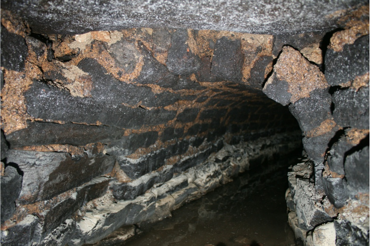
Drain running under Room B8. The masonry lower courses can be dated to c. 1583, while the red brick vault above is dated to a phase of repair in 1720-1740
