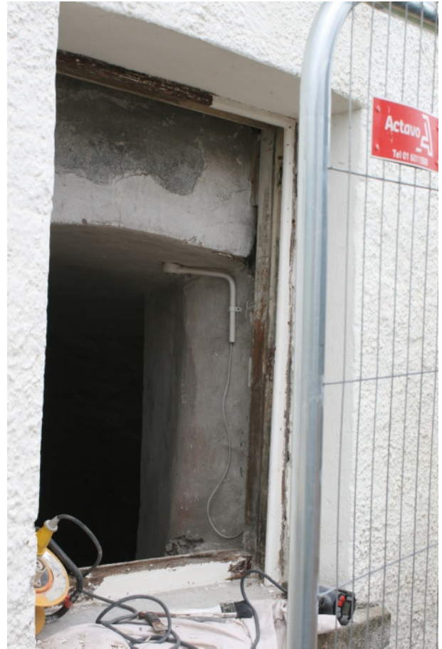
Window of northeast tower (Room B10) from exterior, following removal of Georgian sash window. Note curving ceiling vault on interior of window
