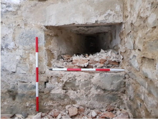
Northern gunloop in tower B10, showing process of removal of brick infill
