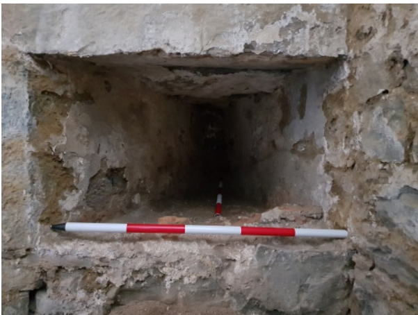
Northern gunloop in tower B10, showing survival of type A clay/loam plaster
