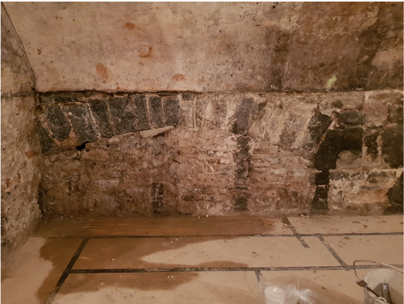
Plaster type C, 18th century lime and aggregate plaster, above springer line in Room B8. The vertical lines of former coal bunkers can be made out below the fireplace voussoirs
