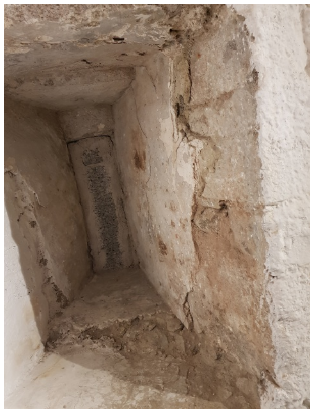
Earth mortar plaster in gunloop at Bagenal's Castle in Newry, Co. Down, constructed in c. 1568-1569
