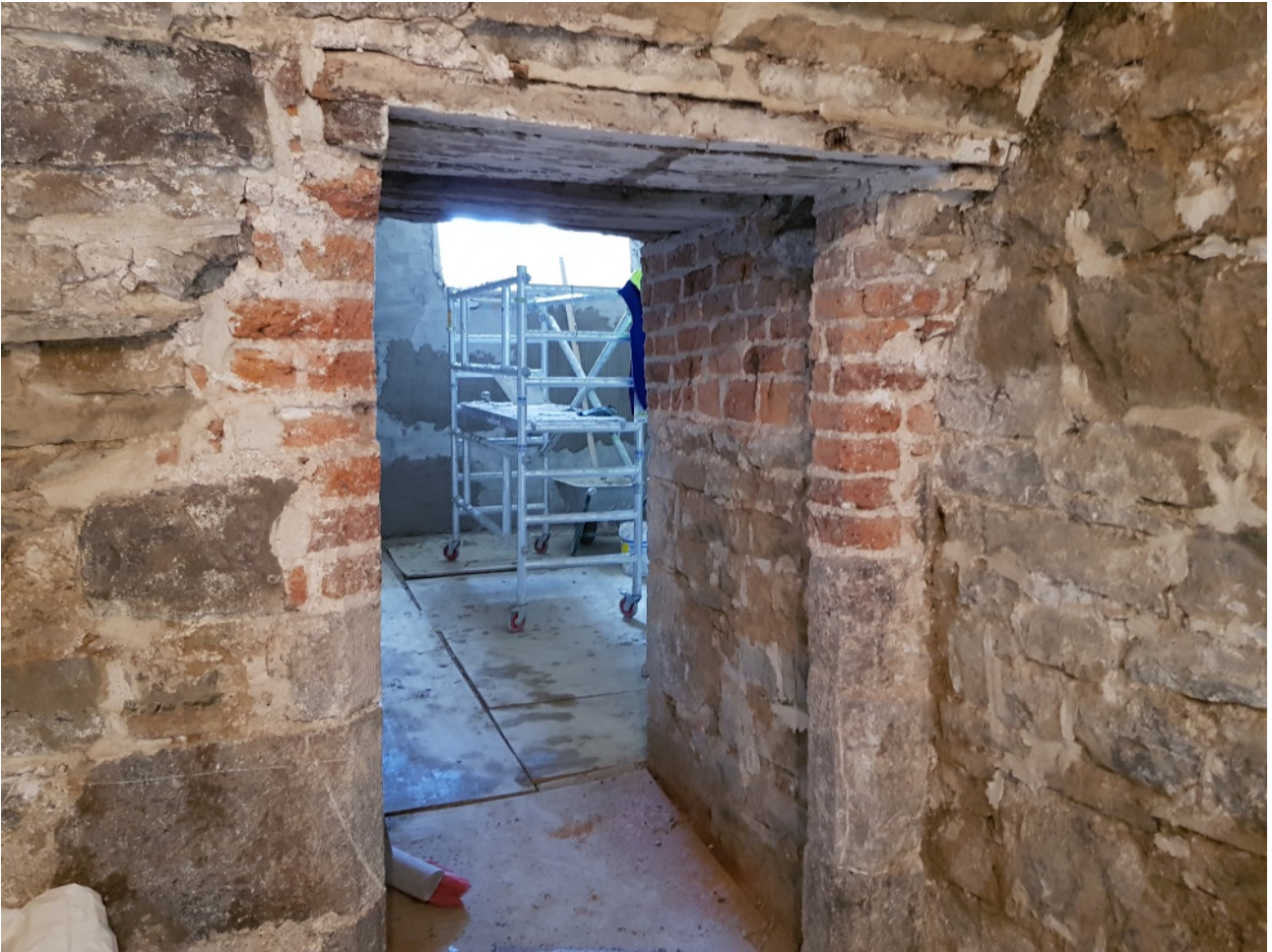
Doorway into northeast tower (B10) showing 16th century stone surmounted by 18th century brick jambs
