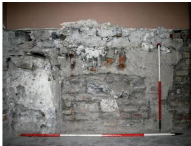
Top: S1 showing possible blocked 18th century window opening Middle: S2 showing top of robbed-out arch for embrasure Bottom: S5 showing lower part of blocked opening
