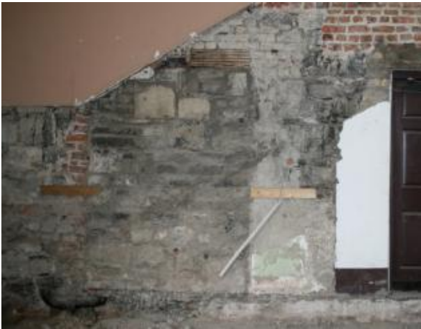
Bottom: W5 showing brick-lined opening, with arched top of opening obscured by scaffolding
