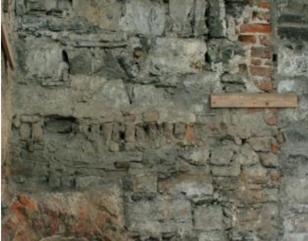
Top: W1 horizontal line of red brick in middle of image, also showing vertical line of red brick to right which is the later opening W2
