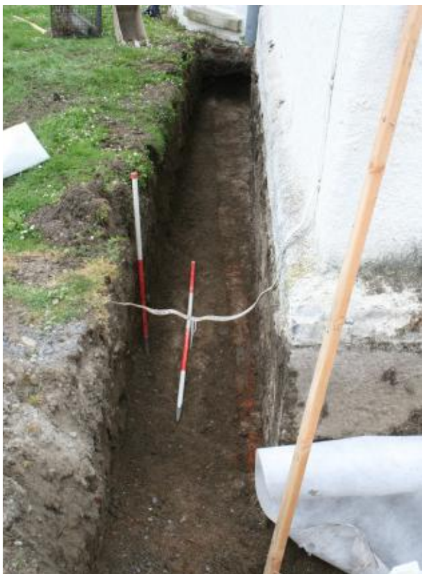
Above: foundations and ground-floor coping identified during the excavations, note how both southern flanker foundations are not squared Below: western foundations of the northeast flanker facing north, showing 18th century red brick cosmetic repair
