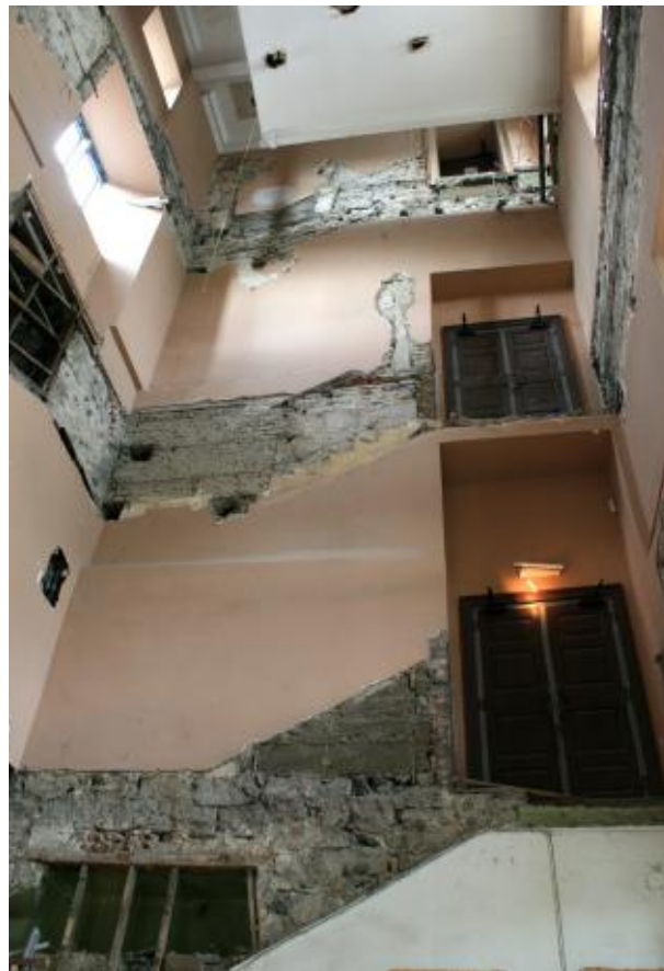
Above: view of north internal wall of flanker. The pink render is 20 th century plaster, and earlier features are visible where this has been removed. The scars of the 20 th century staircase are visible
