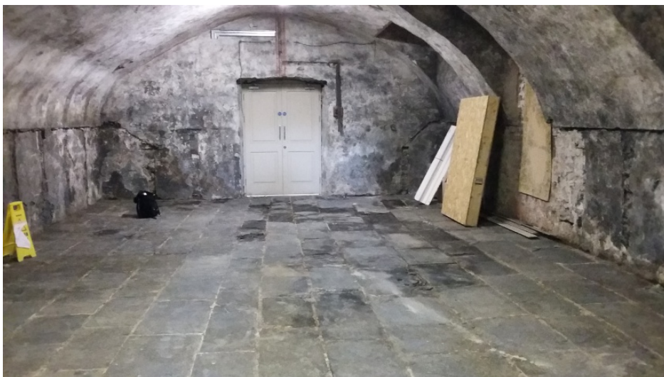
Room B8 facing east, showing 18 th century paved stone floor. Decayed paving stones are darker in colour in centre of photograph.
