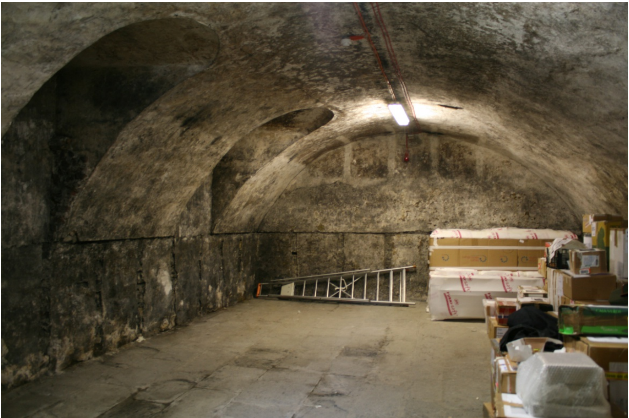
Room B8 facing west, showing partition wall prior to OPW works at rear of photograph
